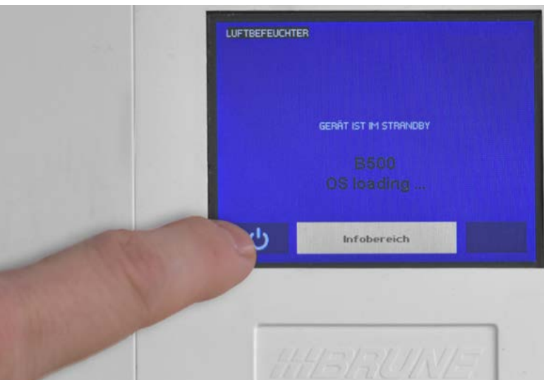
Fig. 4.3.6: Switching on the humidifier
